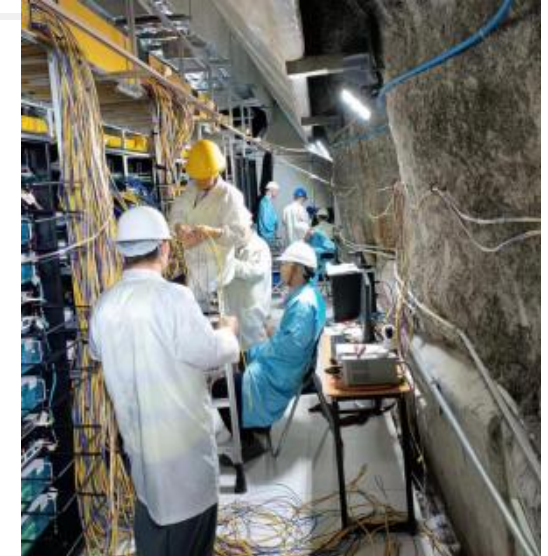
Connected to racks in Electronics room
