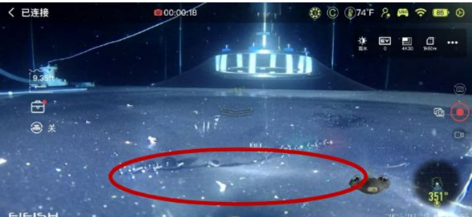
JUNO first crack close to the top chimney,
