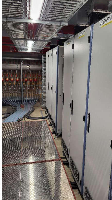
20kW 1300 MHz solid state amplifier modules total 17 modules
