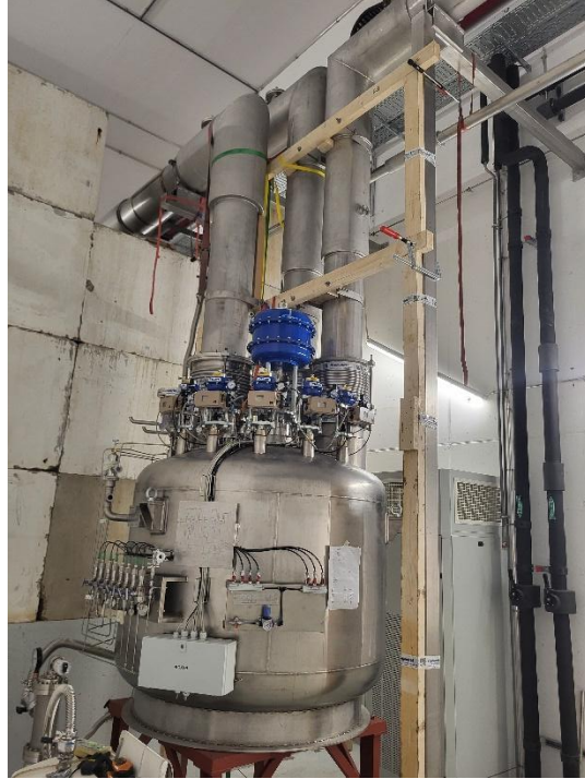
LeHe distribution In central cryobunker (Hall-1)
